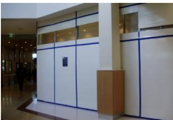
Behind the hoarding work is taking place on the old patient lifts
