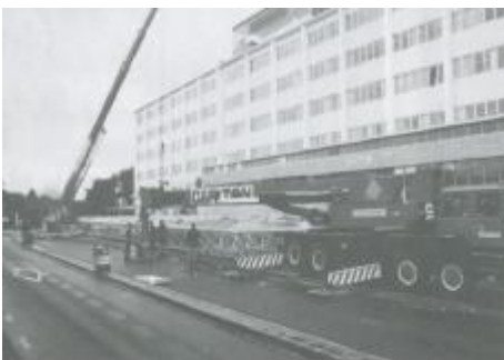
The space frame canopy is about to be lifted on its supports to provide cover for the pedestrian and ambulance entrances to the Emergency Dept.
