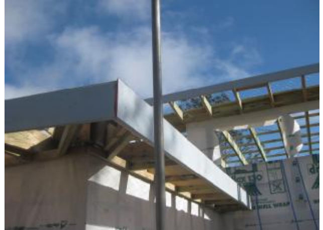
High level window to clinical area. This will attract the natural light.
