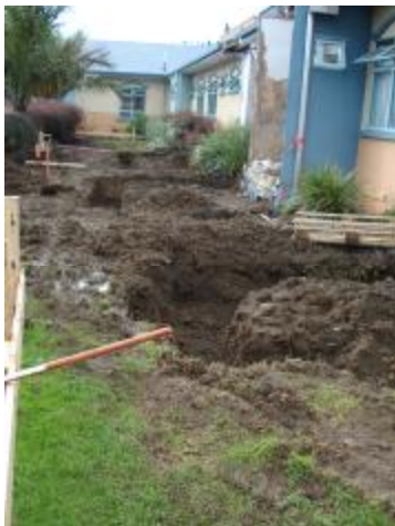
The trenches will form the foundation or base for the ensuite floor slabs and extensions to the two wings.
