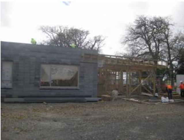
Front of building showing window to ADHB and AUT waiting room and main entrance to all areas.
