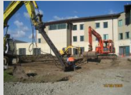
Preparing a screw pile for testing. (The screw piles support the Ground beams and footings).
